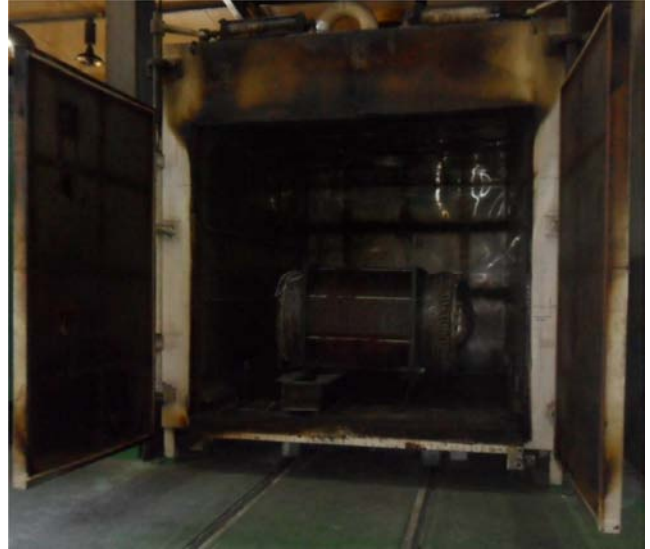
Figure 3. HV motor in drying oven.
